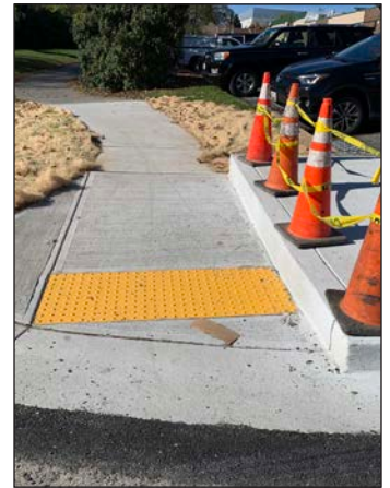
A new curb ramp and sidewalk are installed at the intersection of Ritchie Parkway and Fleet Street connecting to a trail and a nearby shopping center.
