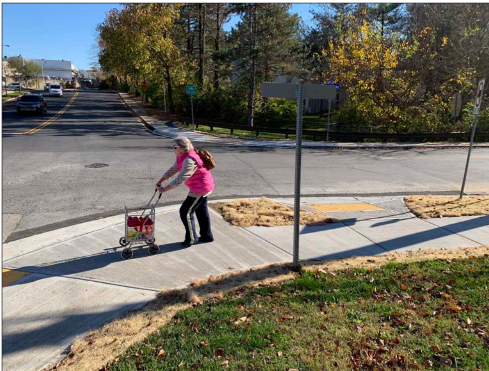
A pedestrian walk along a newly reconstructed sidewalk and curb ramp at Ritchie Parkway and Fleet Street. Photo by City of Rockville.
