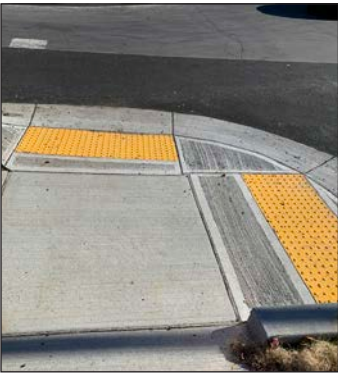
Above: Perpendicular curb ramps are installed at an intersection corner to better direct pedestrians crossing the street.
