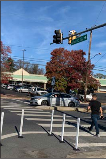
A person crossed Veirs Mill Road (MD 586) at Atlantic Avenue after MDOT SHA installed flex posts to create a curb extension and calm traffic.
